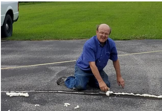
(Left) Gary Vohnout sealing cracks on the runway prior to applying sealant.
